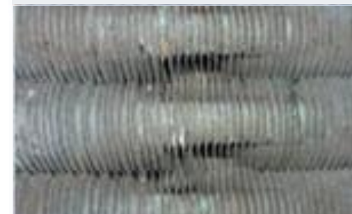
Clean Coil after 3 months
